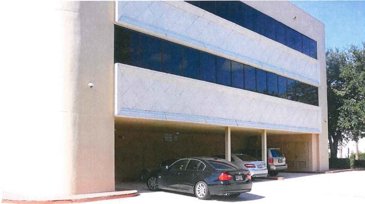
Rear (south) façade – incorporates light colored pre-cast panels with the diamond design
